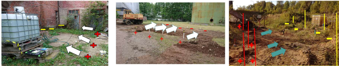
Figure 2.2 a-c. a) Site Villähde, non-saturated zone application b) Site Motala, below ground water level application c) Site Valmiera, non-saturated zone application reaching the ground water level
