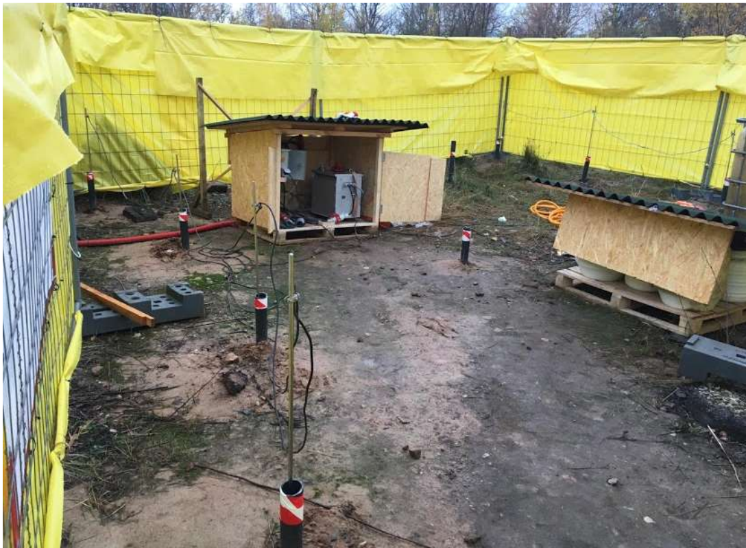
Figure 2.14. Finished site installations. The anode side on the left, the cathode side on the upper right near the fence. Tubes in between mark monitoring sampling spots.
