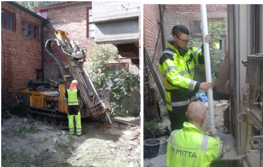
Figure 2.3 a-b. Drilling (a) and installation of perforated tubes (b) at site Nastola in June 2016.
