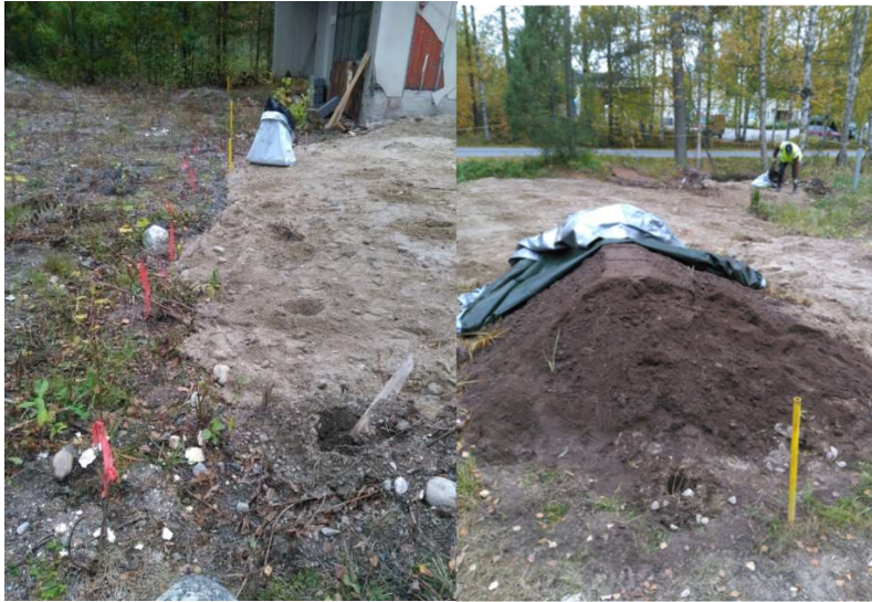
Figure 5.1. Oil and Hb-contaminated hot spots removed by digging before starting the planting.
