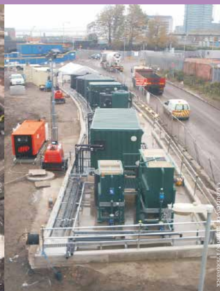
Groundwater treatment works
