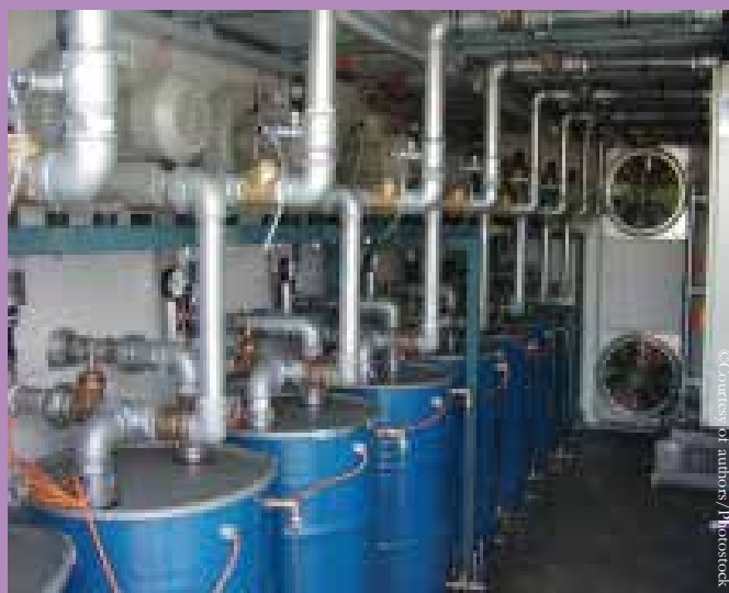
SVE extraction system
