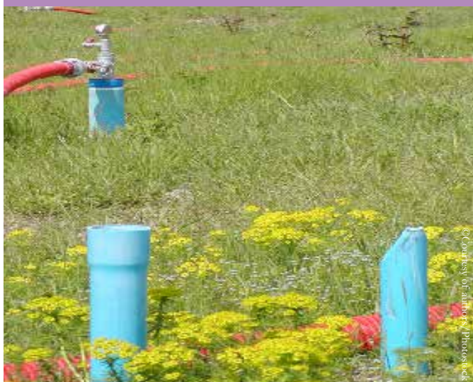
SVE well (with manometer) and two AS wells
