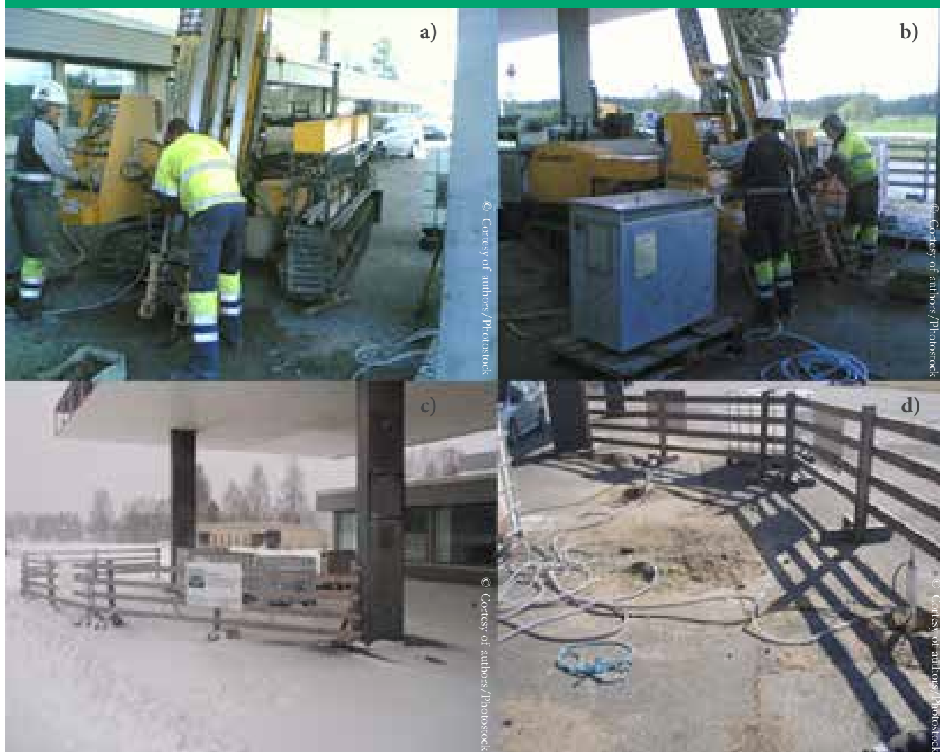
From a-d : a) Jalasjärvi site, b) the installation of perforated tubes and c), d) the electrokinetic in situ treatment.
