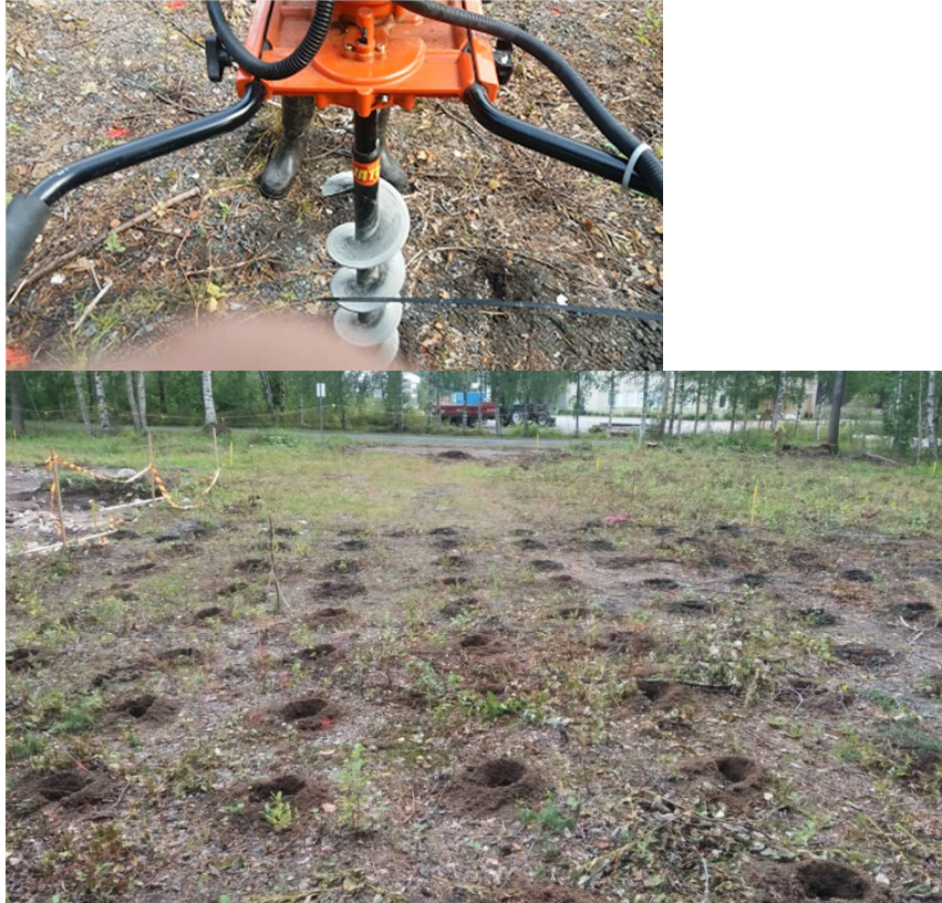
Fig. 6.2. a-b. Drilling holes for planting at the Kiertotie 18 industrial site in Virrat
