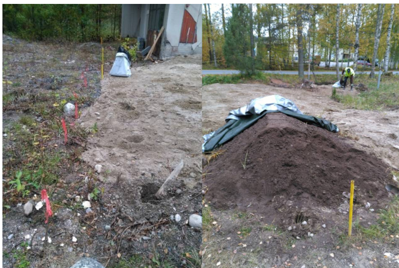
Fig 6.1. Oil and Hb-contaminated hot spots removed by digging before starting the planting
