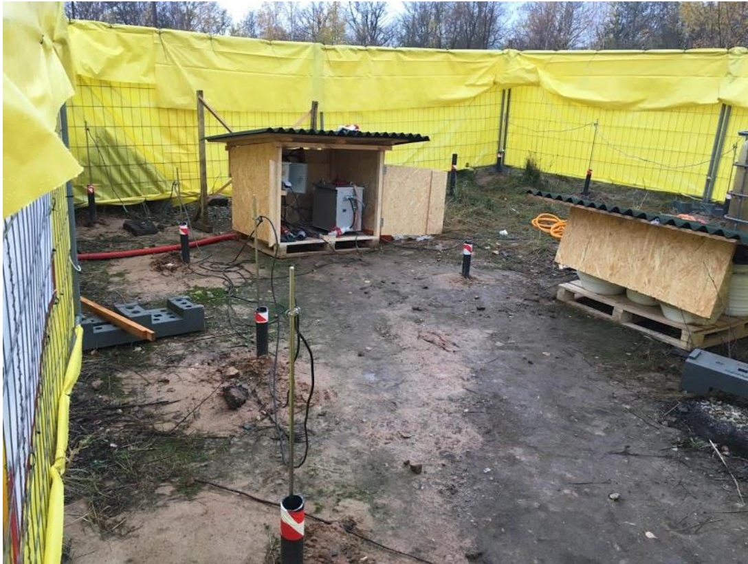
Fig. 3.2. Finished site installations. Anode site on the left, cathode site on the upper right near fence. Tubes in between mark alternative sampling spots.
