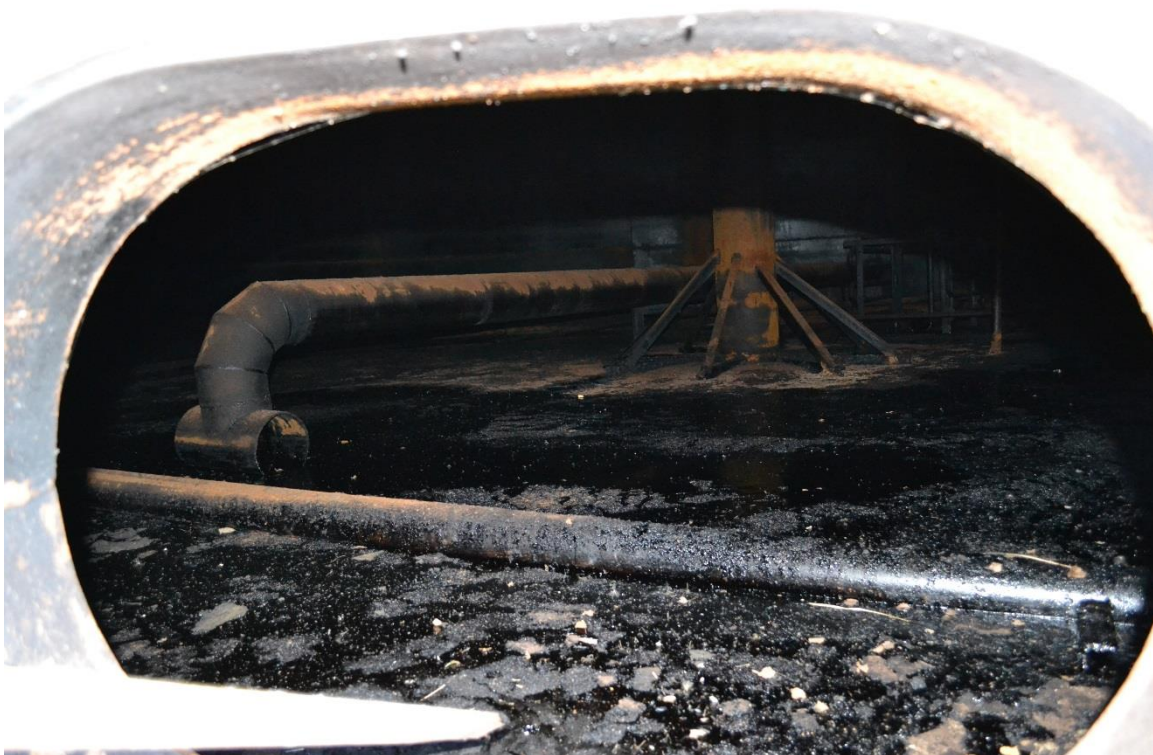
Figure 3. Remains of semi-liquid black fuel in the bottom of reservoir (photo from site visit in October, 2016)
